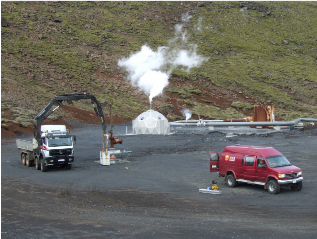
FIGURE 3: Logging of a high temperature well
