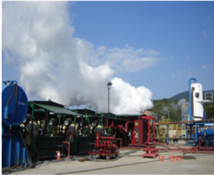
FIGURE 5: Test of the production of a geothermal well with compressed air equipment for aerated drilling
