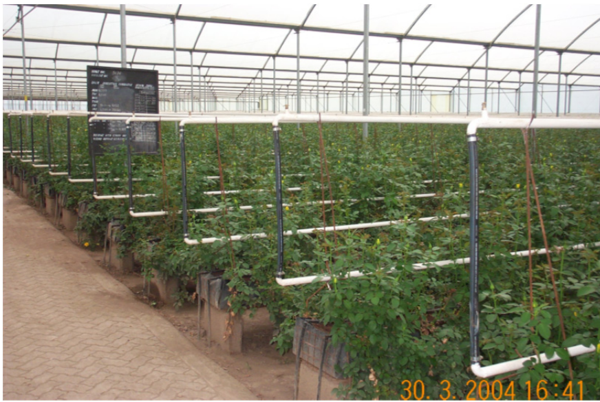
FIGURE 4: Greenhouse heating at Oserian Development Company, Naivasha, Kenya
