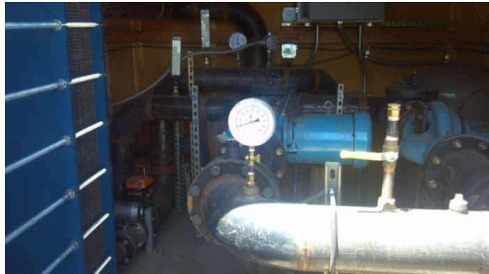
FIGURE 2: Klamath Falls heat exchange building. Some of the clients of the hot city water are 24 commercial and government buildings, greenhouses, sidewalk snow melt and a beer brewing company (Chiasson, 2006)
