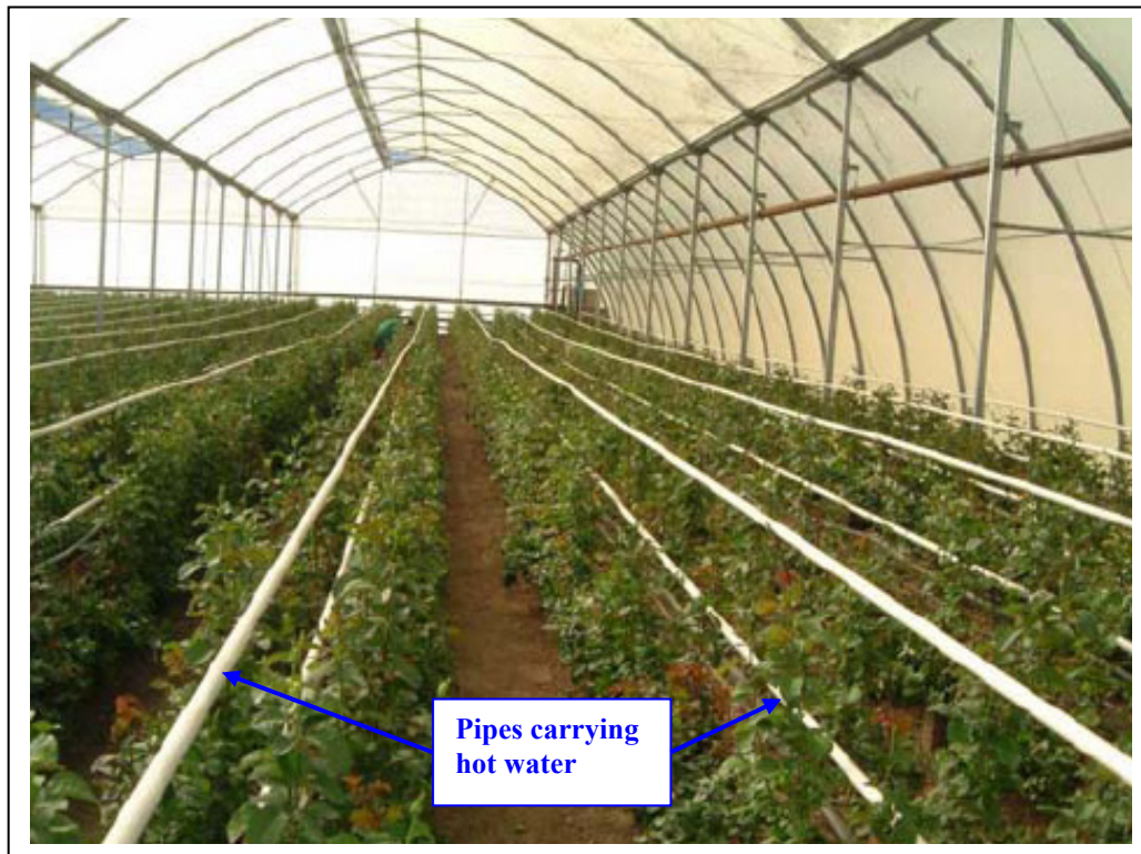
FIGURE 6: Geothermal greenhouse heating at Oserian Company, Kenya.
