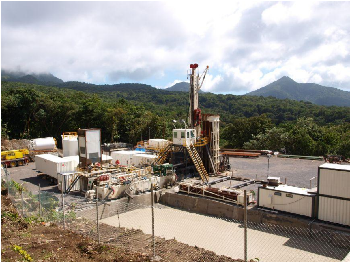
FIGURE 1: Rig (100 t) drilling a slim hole to 1500 m with 7" production casing and a 4½" slotted liner
