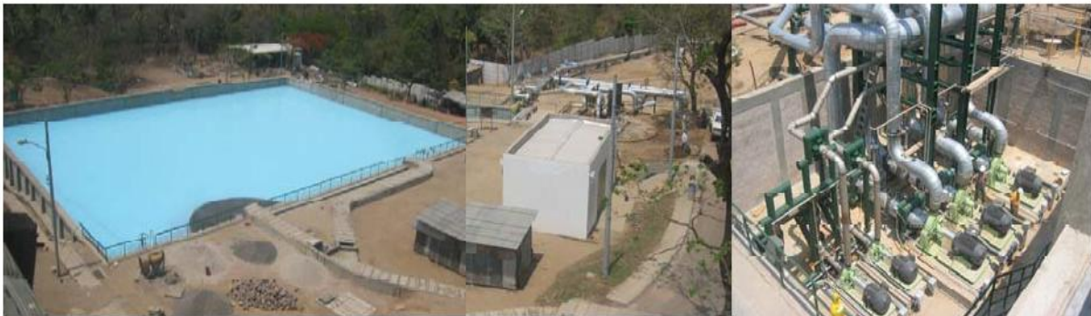
FIGURE 5: Pumping station for brine injection in Ahuachapán
