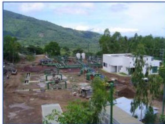
FIGURE 9: Pumping station in well pad TR-1
