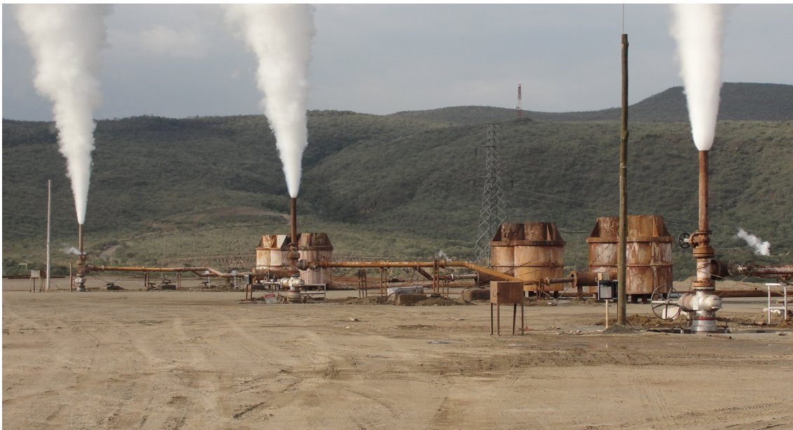
FIGURE 8: Wells discharging at OW- 44 at Olkaria East Field with silencers to abate noise levels
