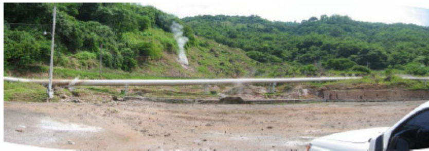
FIGURE 13: El Tronador Fumarolic area with steam gathering system near the Berlin power plant. A long gabion wall was built on the southern flank of the pipeline
