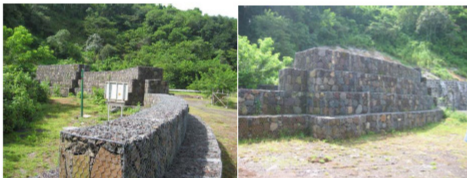
FIGURE 9: Gabion wall at TR2 as seen from the east side. The dam is built in sections, 2, 4, and 5 m high, as seen on the picture. b) The gabion wall seen from the north side
