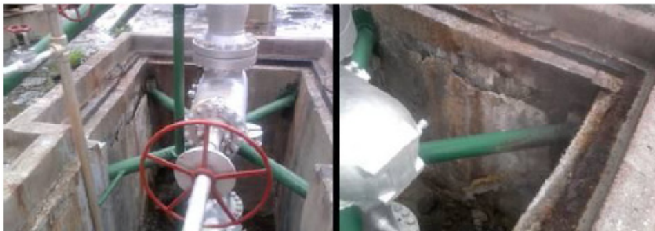
FIGURE 6: Damages on the cellar, well TR-2. Hydrothermal manifestations in the northern corner
