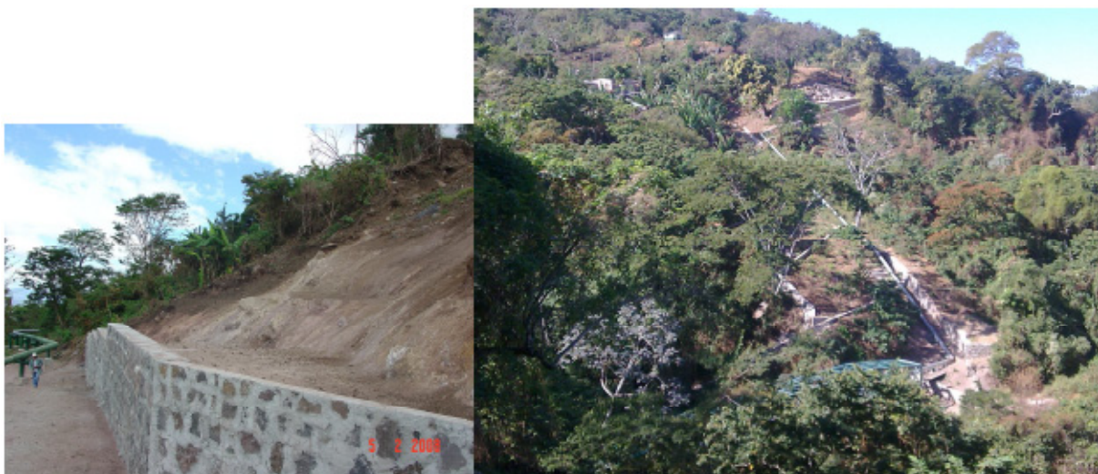
FIGURE 14: a) Mitigation works on the northern slope of the gathering system TR17s/TR18's to injection well TR19's after a landslide occurred in the year 2007. b) Gathering system along the slope close to TR19 injection well
