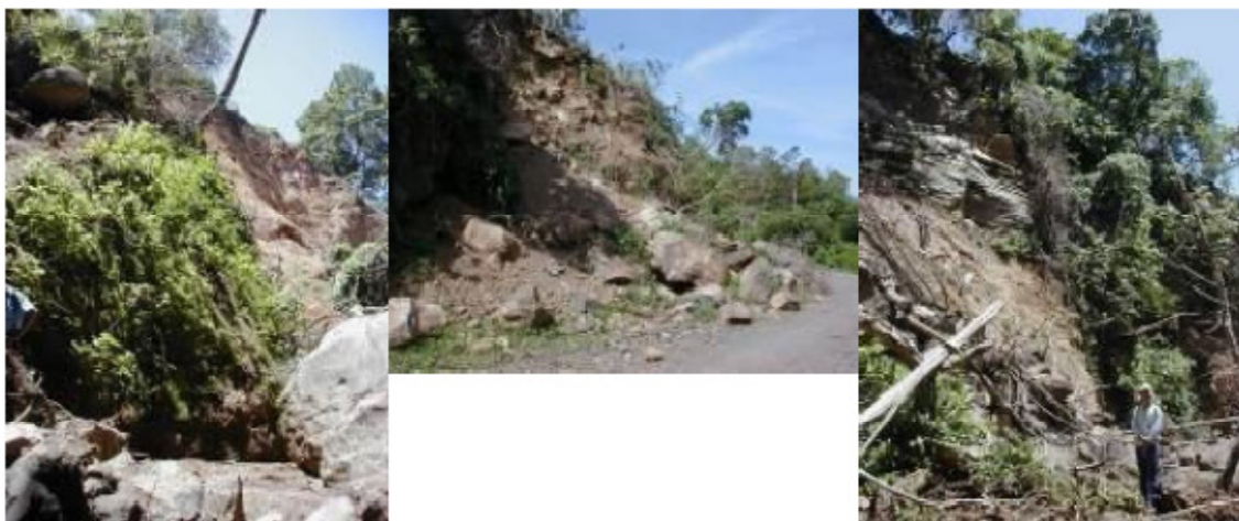
FIGURE 4: Several rock falls located a) West of TR4, Berlin Field, b) Road Mercedes Umaña-Berlin City, c) West of well TR11, occurred during the two earthquakes in January 13 th and February 13 th 2001.
