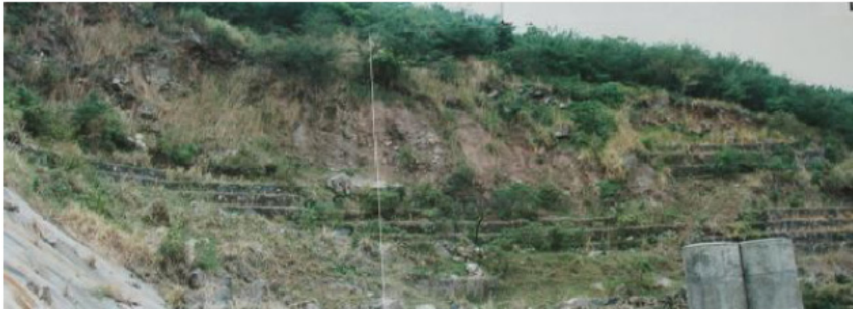
FIGURE 8: Western slope of platform TR2 in the year 1990-1991; several gabion walls were built
