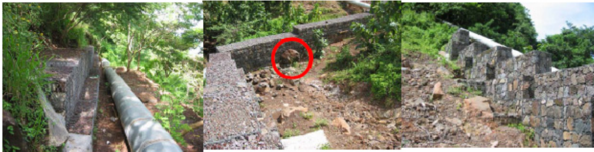
FIGURE 12: a ) The gabion wall is adjusted and not leaning against the pipeline. b) The gabion wall is built to secure the pipeline (following the outer side of the wall) against slides. A rock fall has already hit the wall (red circle), without making any signs of destruction. c) The gabion wall along the pipeline down slope seems sufficient to prevent new damages from slides. The fundamentals of the pipeline were partly damaged in a previous slide
