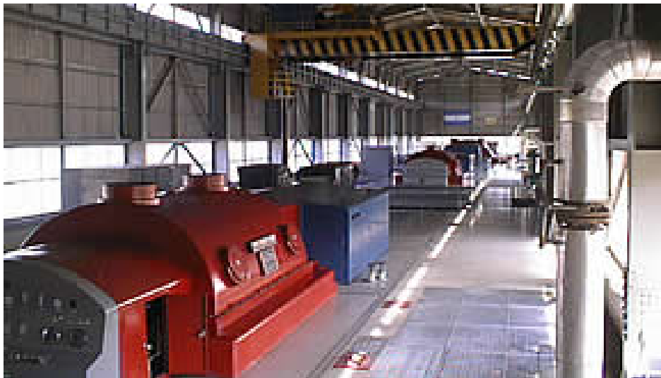
FIGURE 7: Machinery room in Ahuachapan power plant
