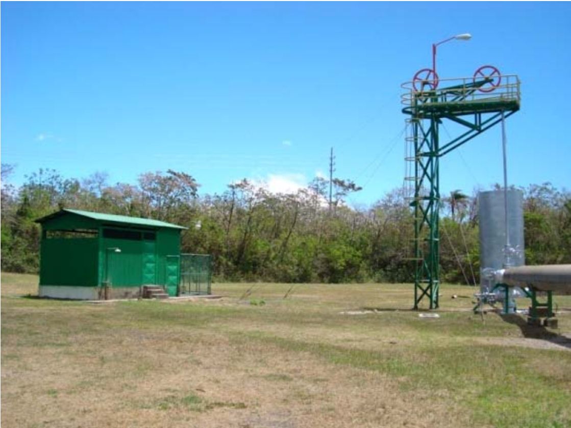
FIGURE 5: The calcium carbonate inhibition system at well PGM-03 (Photo by P. Moya)
