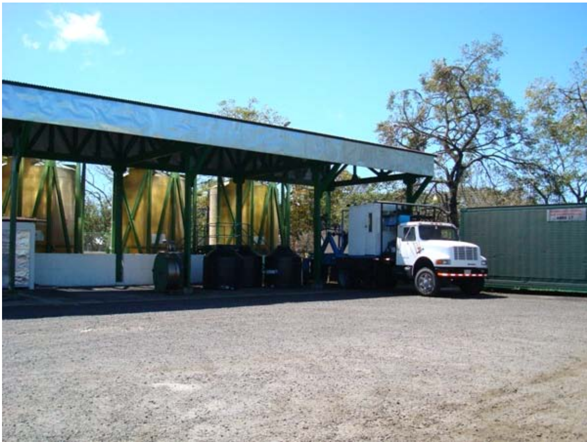
FIGURE 7: Dilution plant at the Miravalles geothermal field (Photo by P. Moya)
