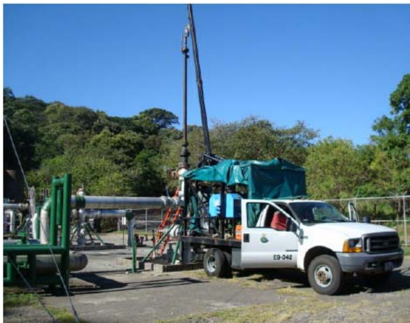
FIGURE 3: Surveys run into a production well, TR-4C, Berlin geothermal field
