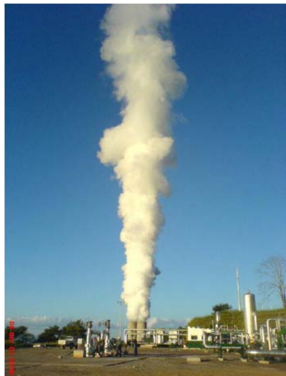
FIGURE 1: Well TR-18 discharged to the mufflers system before being derived into separation station, Berlin geothermal field
