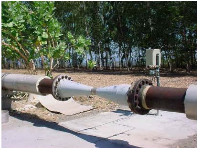
FIGURE 4: Measurement element installed in the pipe for reinjection (Venturi)
