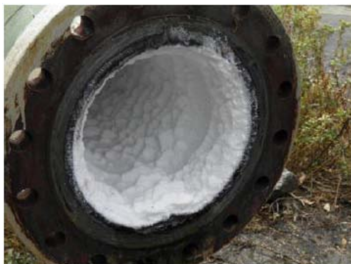
FIGURE 5: Silica deposition found inside the pipe to reinjection well
