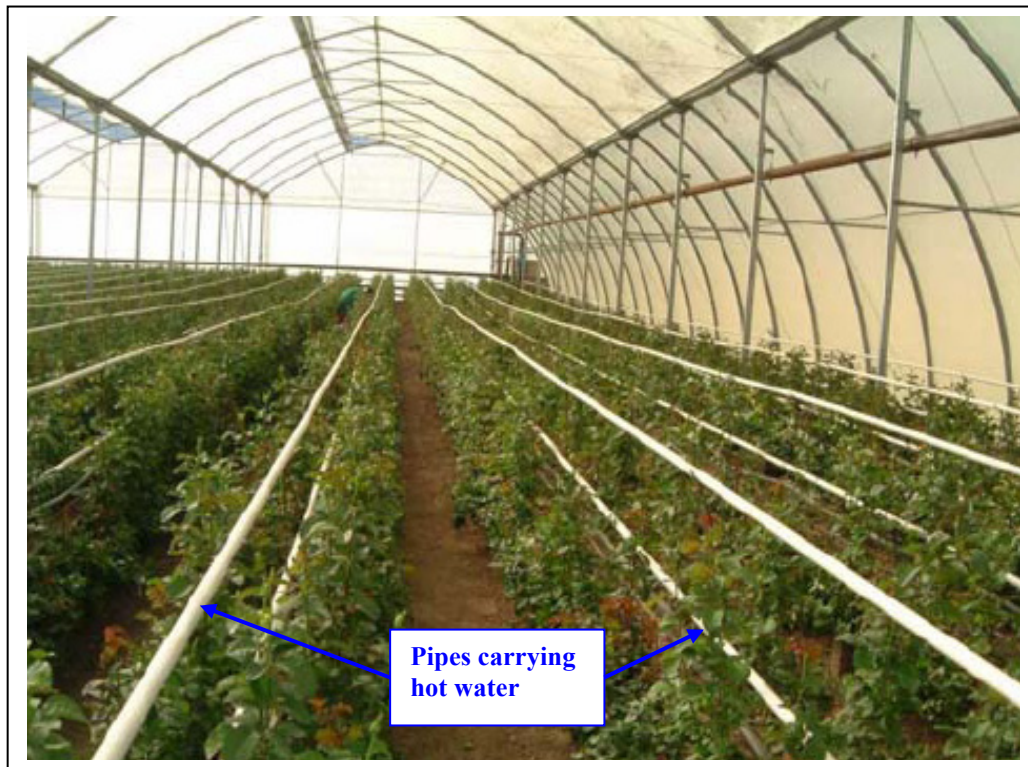
FIGURE 6: Geothermal greenhouse heating at Oserian Company, Kenya.
