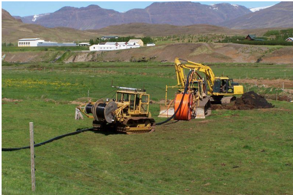
FIGURE 15: Black pipe on the grass is the plastic district heating pipe and the bulldozer carry reels of electrical cables and orange reel is for the fibre optic cable. The bulldozer in the back has the plough that installs all of the pipes simultaneously.
