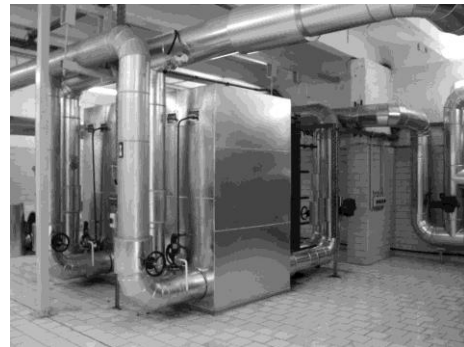
FIGURE 14: Geothermal plant in Neubrandenburg after retrofitting
