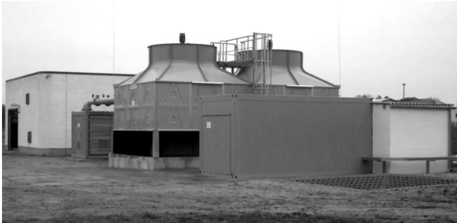
FIGURE 10: ORC unit at the Neustadt-Glewe site
