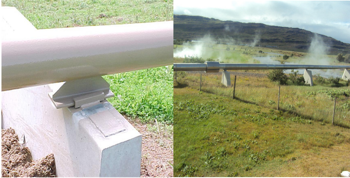
FIGURE 6: Horizontal supports on the left and pipe supports on the right
