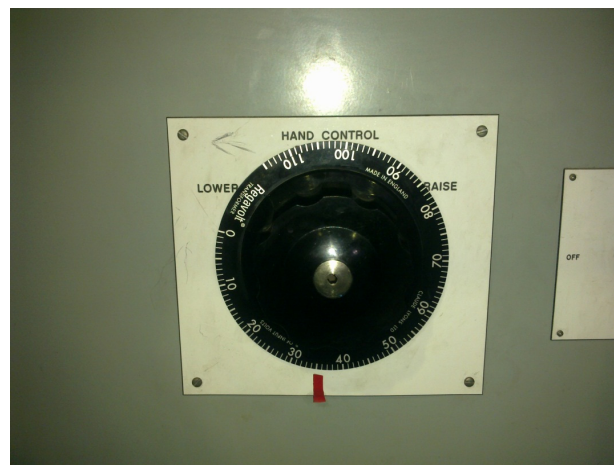
FIGURE 7: Generator 6 manual power factor control
