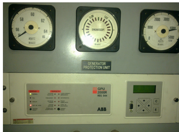
FIGURE 5: Generator 7 numerical protection relay
