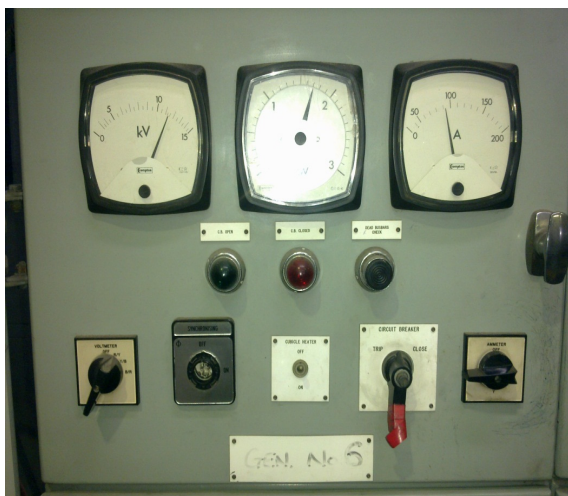
FIGURE 6: Generator 6 analogue power parameter displays
