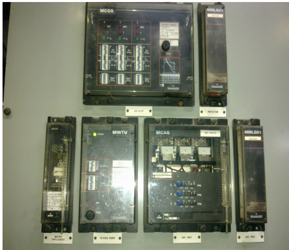
FIGURE 4: Generator 6 static protection relays
