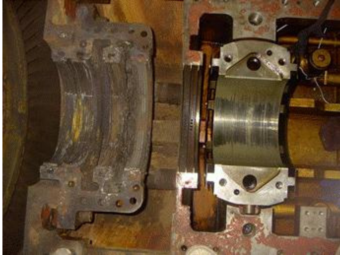
FIGURE 2: Seal damage due to scaling
