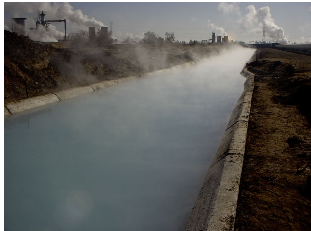
FIGURE 1: Higher water level in channels due to scaling
