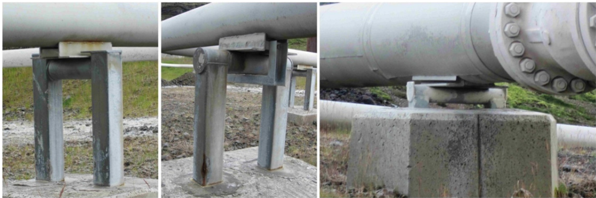
FIGURE 10: From left to right, horizontal and vertical pipe supports (pictures are taken from Nesjavellir Geothermal Power Station)
