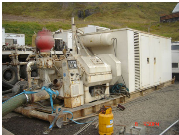
FIGURE 10: Mud pump and tank. Note soundproofing enclosure
