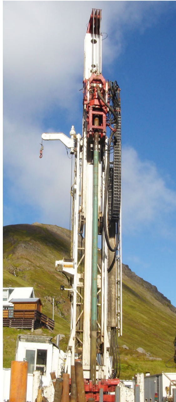
FIGURE 7: Mast and top drive
