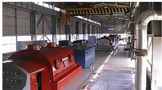
FIGURE 7: The machinery room in the Ahuachapan power plant
