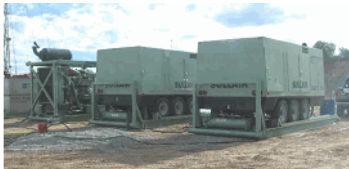
FIGURE 3: The air compressor
