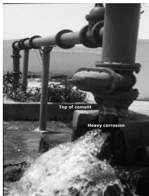
FIGURE 4: Wellhead of Sai with corrosion
