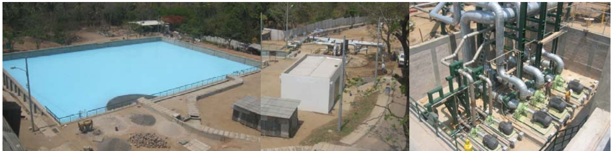
FIGURE 11: Pumping station for brine injection in Ahuachapán
