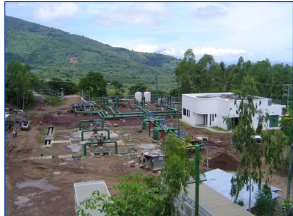
FIGURE 14: Pumping station in wellpad TR-1
