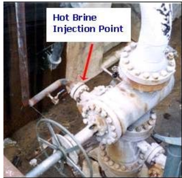
FIGURE 5: Hot brine wellhead washing
