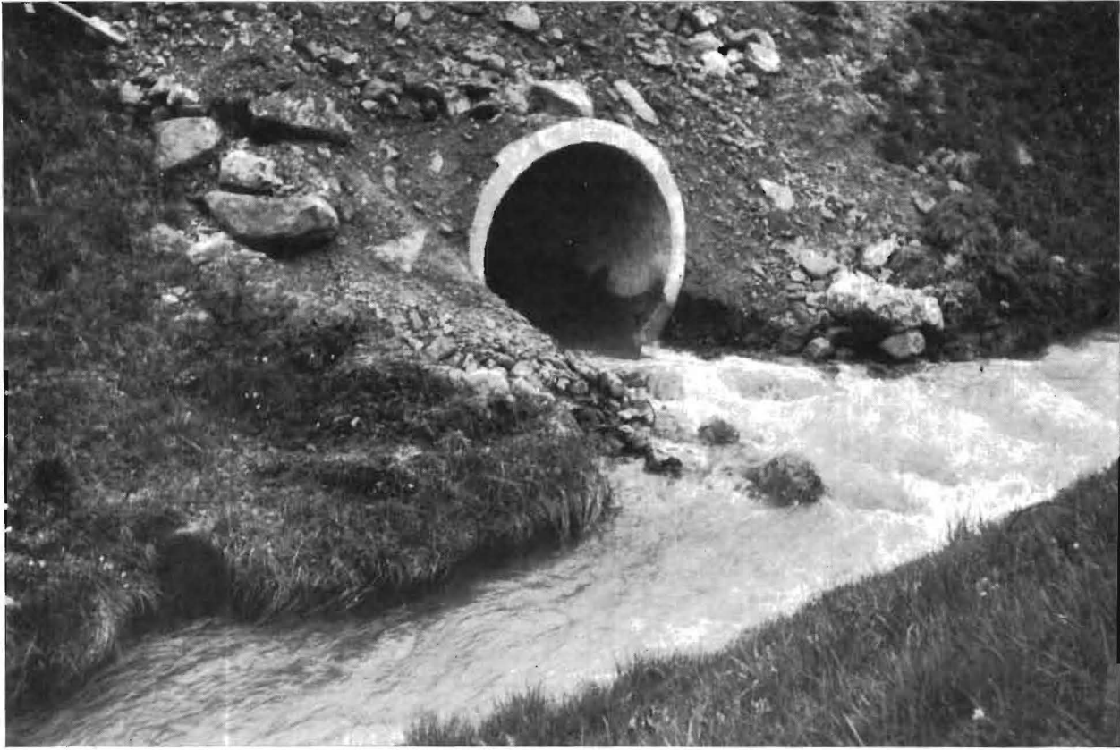
Fig. 50 Underground stream passage under Swiss Highway N 3
