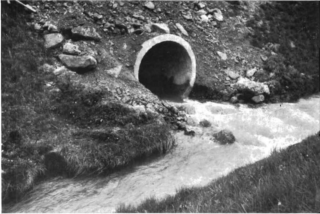
Fig. 50 Underground stream passage under Swiss Highway N 3
