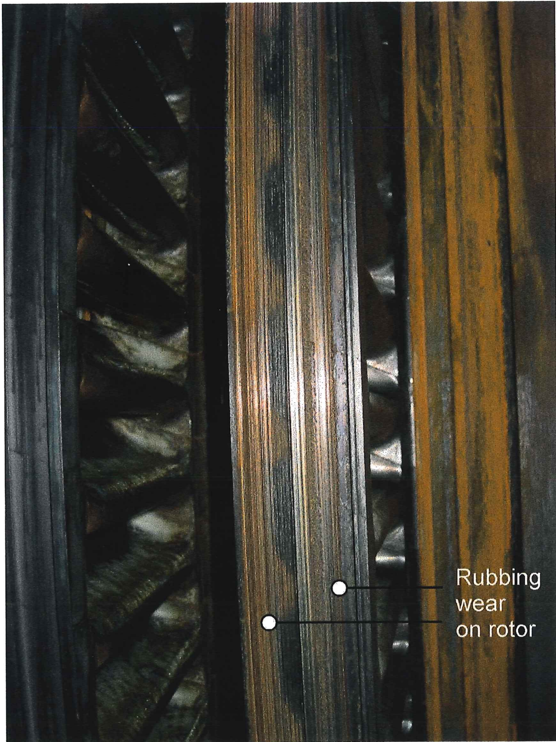
Figure 5. Rotor wear on 1 st stage shroud opposite the sealing fins where sample #2 is taken. Photograph taken after initial high-pressure water washing of turbine rotor.
