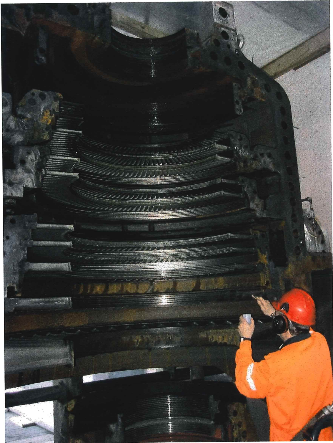
Figure 6. Upper half of turbine casing after initial high-pressure water washing. No deposition was remaining that could be removed for analysis.
