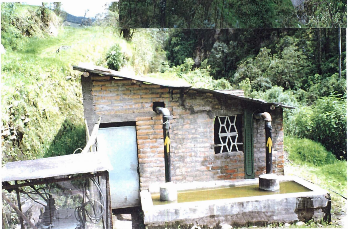
Picture 18. Booster pump 1. Note concrete header on suction side (also on discharge side).
