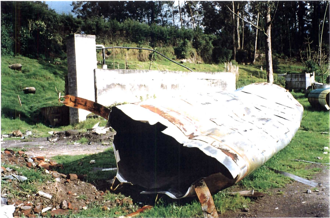
Picture 13. Concrete separator of Alborada A. Collapsed separator tank in foreground.
