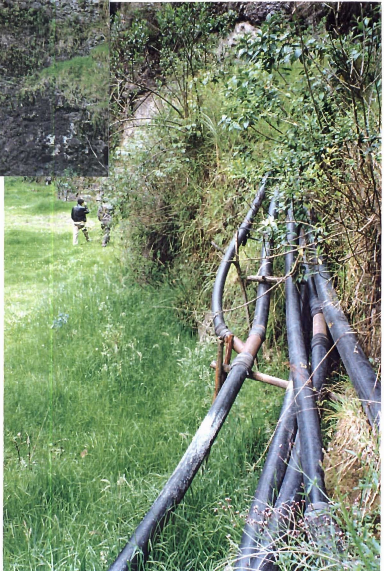
Picture 10. The HDPE gas collection pipelines from booster station 1, close to Tatatambo
